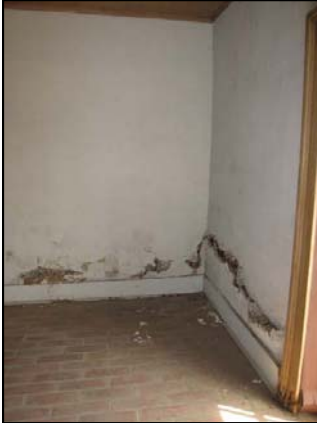
Figure 55: Detail of cracked wall (CA, 2009)
