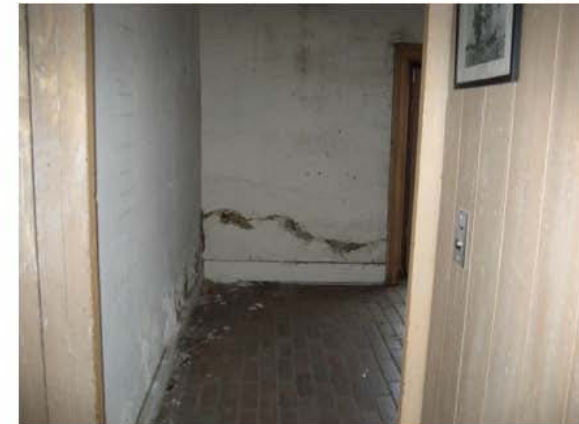
Photo 5 - Brick floor. Water damage on wall. This is caused by moisture rising from the ground.
