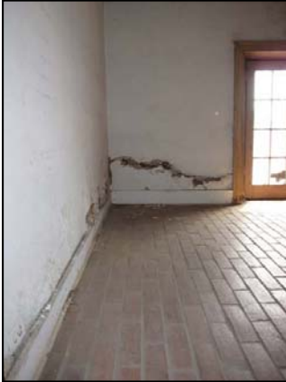
Figure 54: Interior of south wing, east elevation (background), note cracked wall (CA, 2009)
