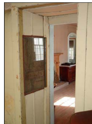
Figure 48: Connection between north and south wings, note panel removed to reveal adobe construction, view south-east (CA, 2008)
