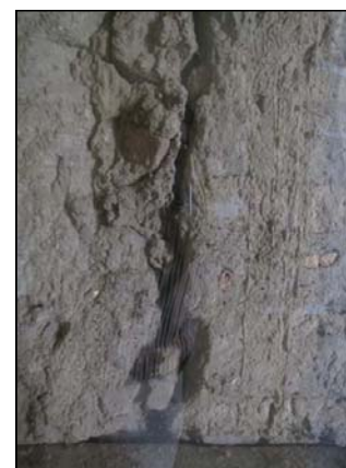
Figure 49: Detail of adobe construction, view east, note north wing wall (left) and south wing wall (right) with gap (CA, 2009)
